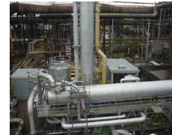
Steel Plant (Japan)
